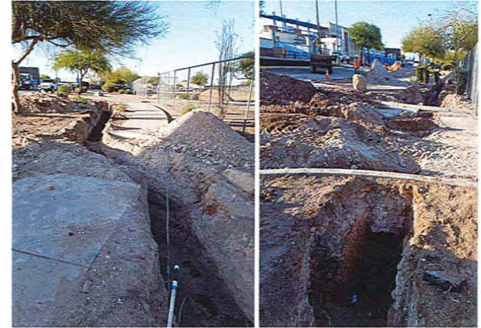
Pima County Kino Sports Complex & Stadium District Project Infrastructure to deliver reclaimed and collected stormwater – saving 30 acre-feet of potable water, annually – the equivalent of 90 households
