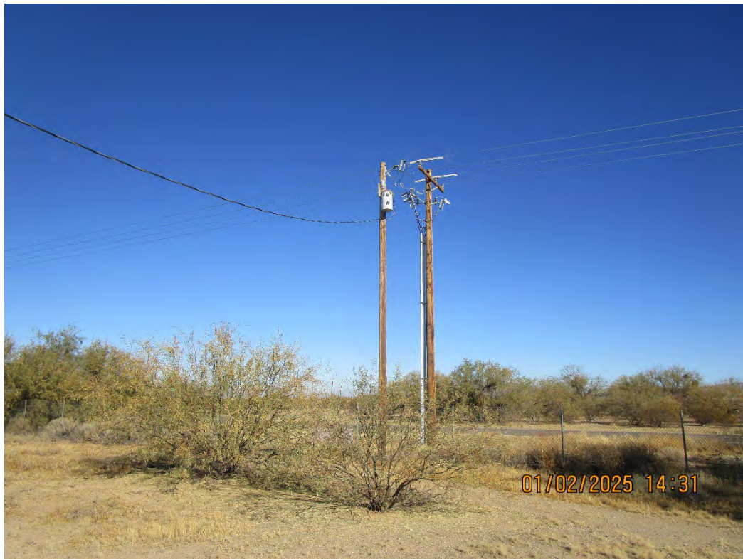
View of existing electrical facilities serving property and proposed site.
