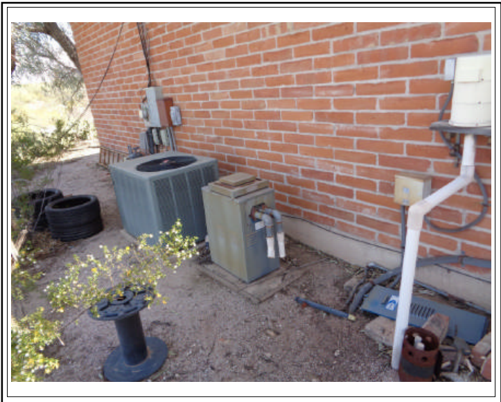
ELECTRICAL SERVICE ENTRY POINT, REFLECTING AN UPDATED HVAC SYSTEM.
