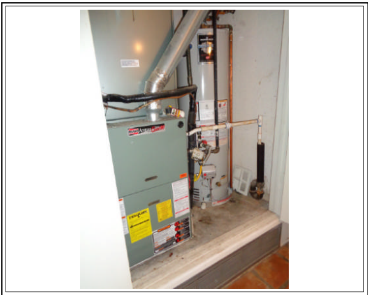
MECHANICAL, ALSO REFLECTING UPDATED HVAC AND WATER HEATER, TO INCLUDE SOME PLUMBING LINES
