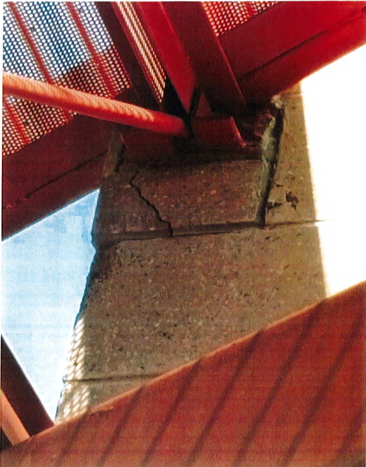
Photo of Item #3 Exterior Walls - Needs Attention
