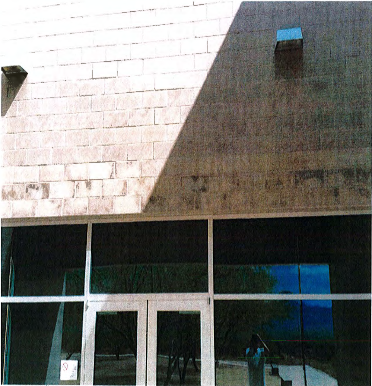
Photo of Item #3 Exterior Walls Needs Sealed - Needs Attention
