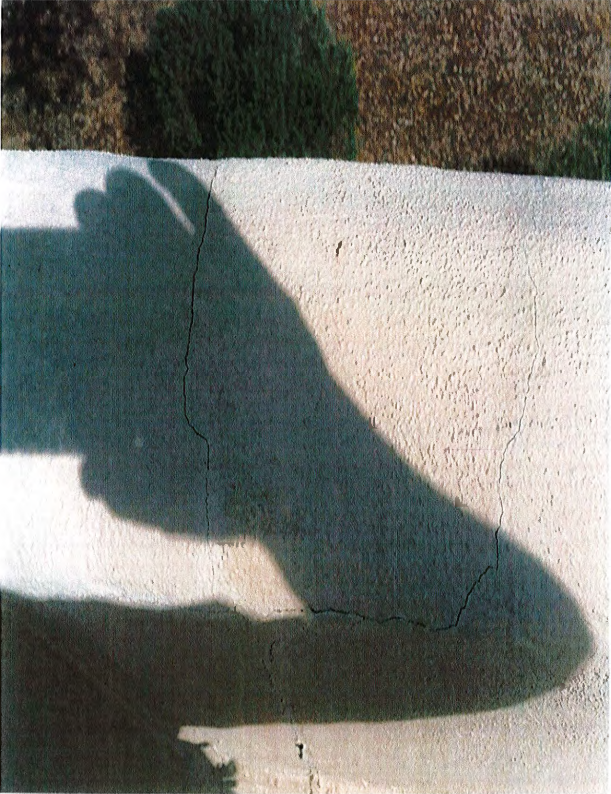
Photo of Item #21 Parapet Roof Fracture - Needs Attention
