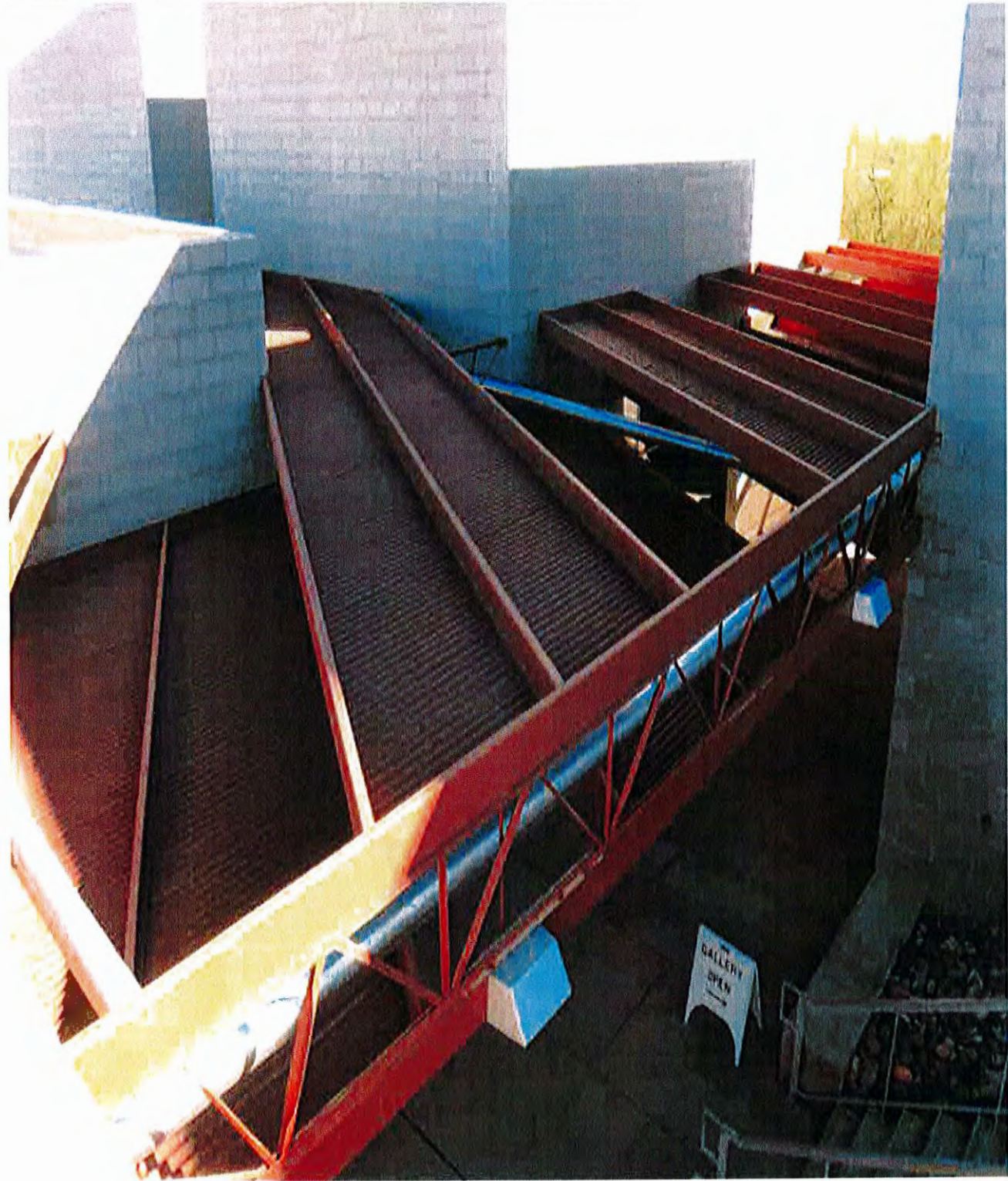
Photo of Item #3 Exterior Walls Needs Sealed - Needs Attention
