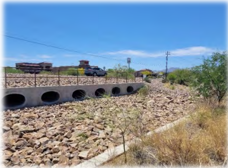
Julian Wash drainage structure under Colossal Cave Road that touches southeast property
