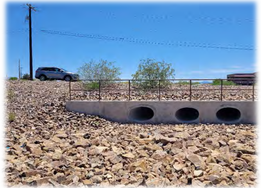
Julian Wash drainage structure under Colossal Cave Road that touches southeast property corner
