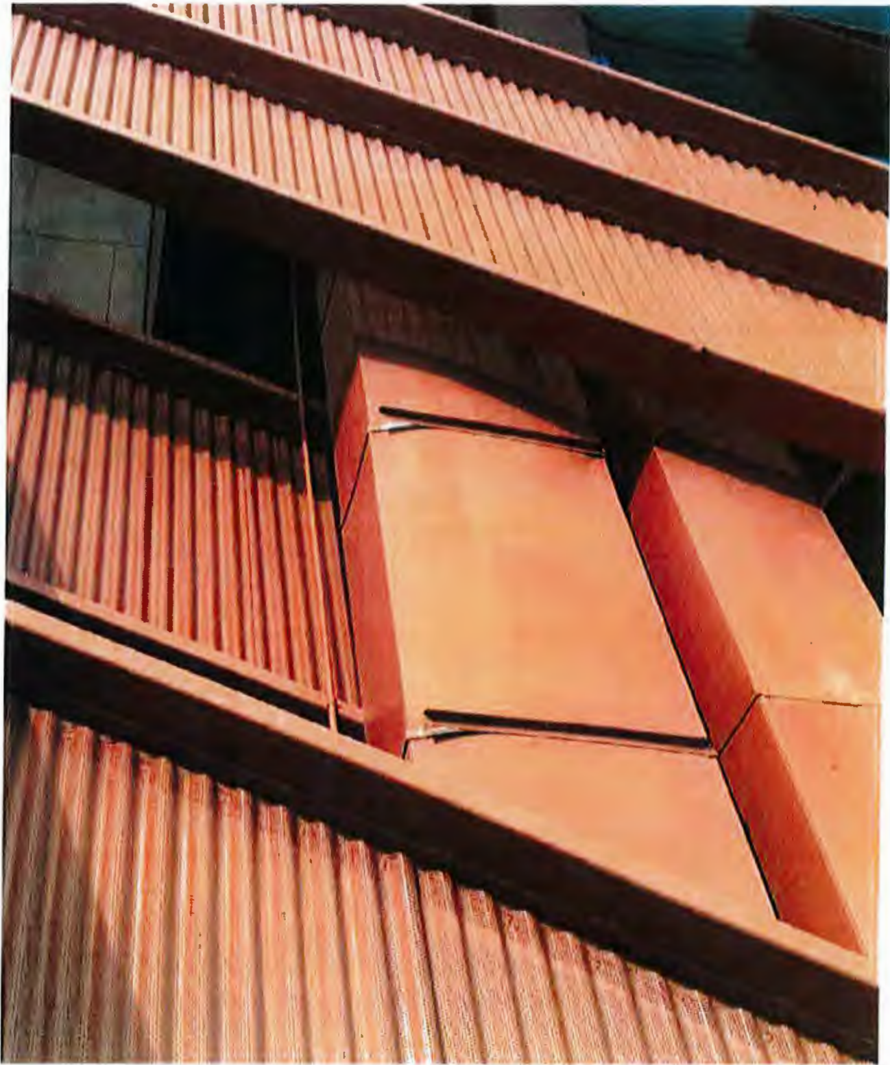
Photo of Item #20 Exterior Duct Work Needs Attention
