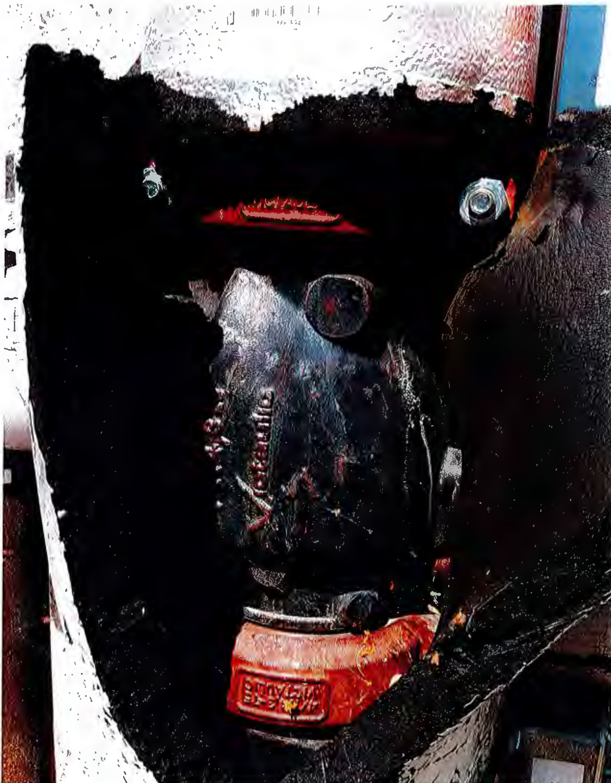
Photo of Item #12 Close Up of Fire Riser South End - Needs Attention
