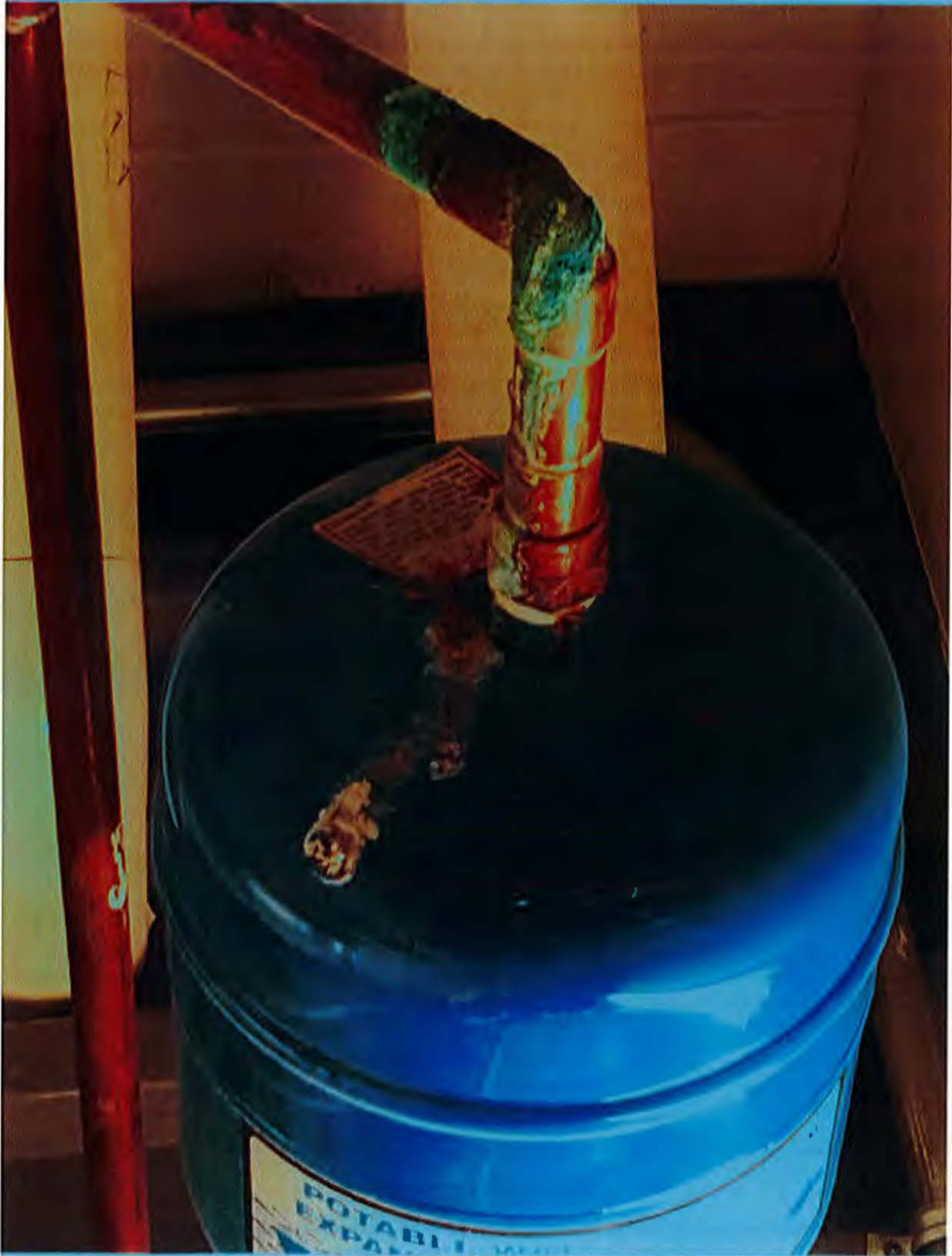
Photo of Item #10 Rheem Water Heater Model 81VP10S - Needs Attention
