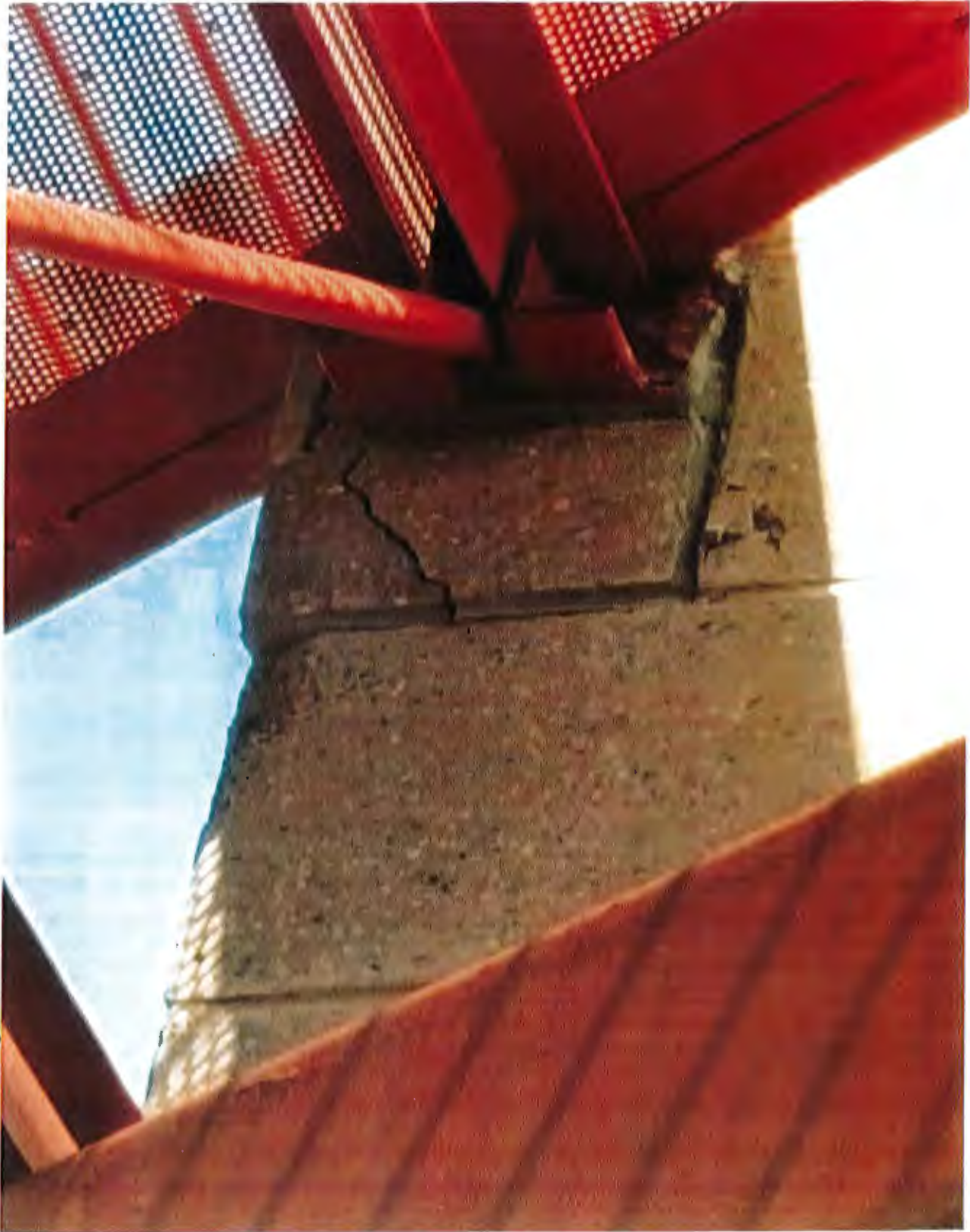
Photo of Item #3 Exterior Walls - Needs Attention
