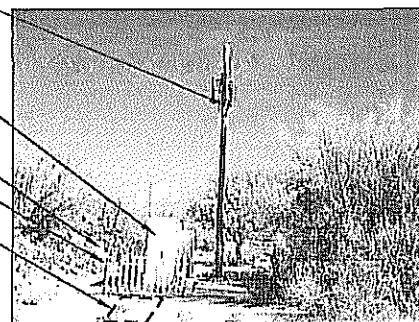
VIEW OF NEW GENERATOR LOCATION (WEST VIEW)
